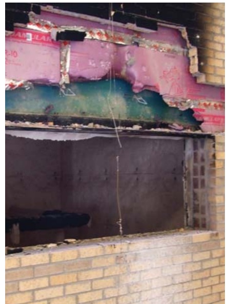
FOAMULAR® XPS with brick veneer stripped away above the test window showing limited damage and minimal fire spread after the NFPA 285 fire test.
