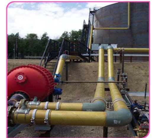
High Pressure Pipe
